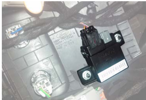
DO NOT DISCONNECT! The PCM Module controls the keyless entry and once disconnected has to be reset by manufacturer. Unsecure from OEM trim and set back out of the way.
